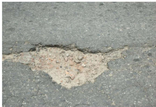
Fig.3. Potholes on Road
