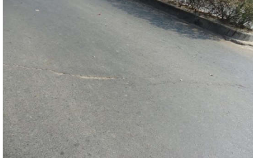
Fig.1. Transverse Cracking on Road
