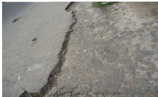
Fig.6. Rutting on Road
