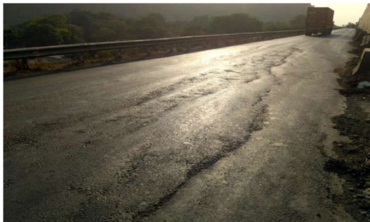
Fig. 1 Cracking along the road in traditional method
